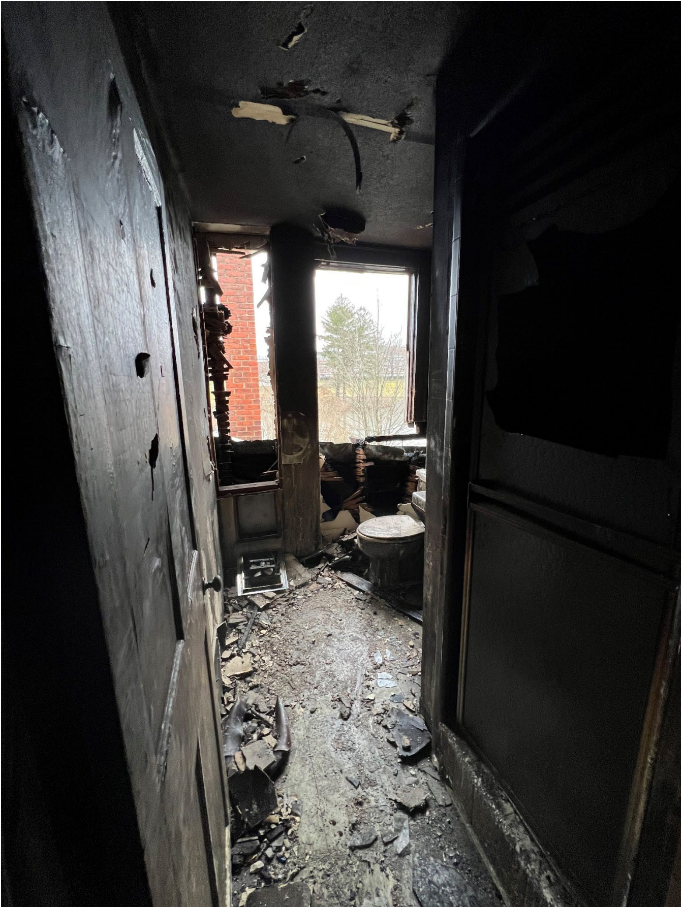
Interior Fire Damage
