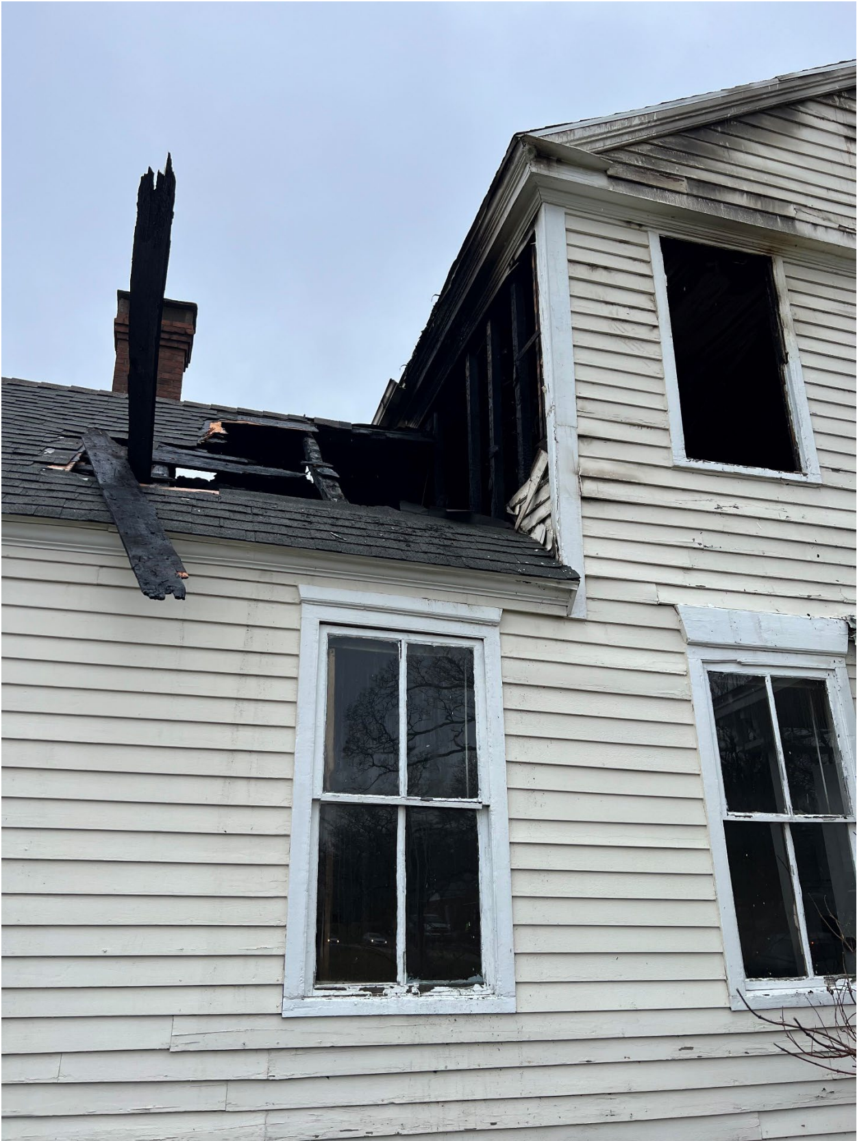
Fire Damaged Roof
