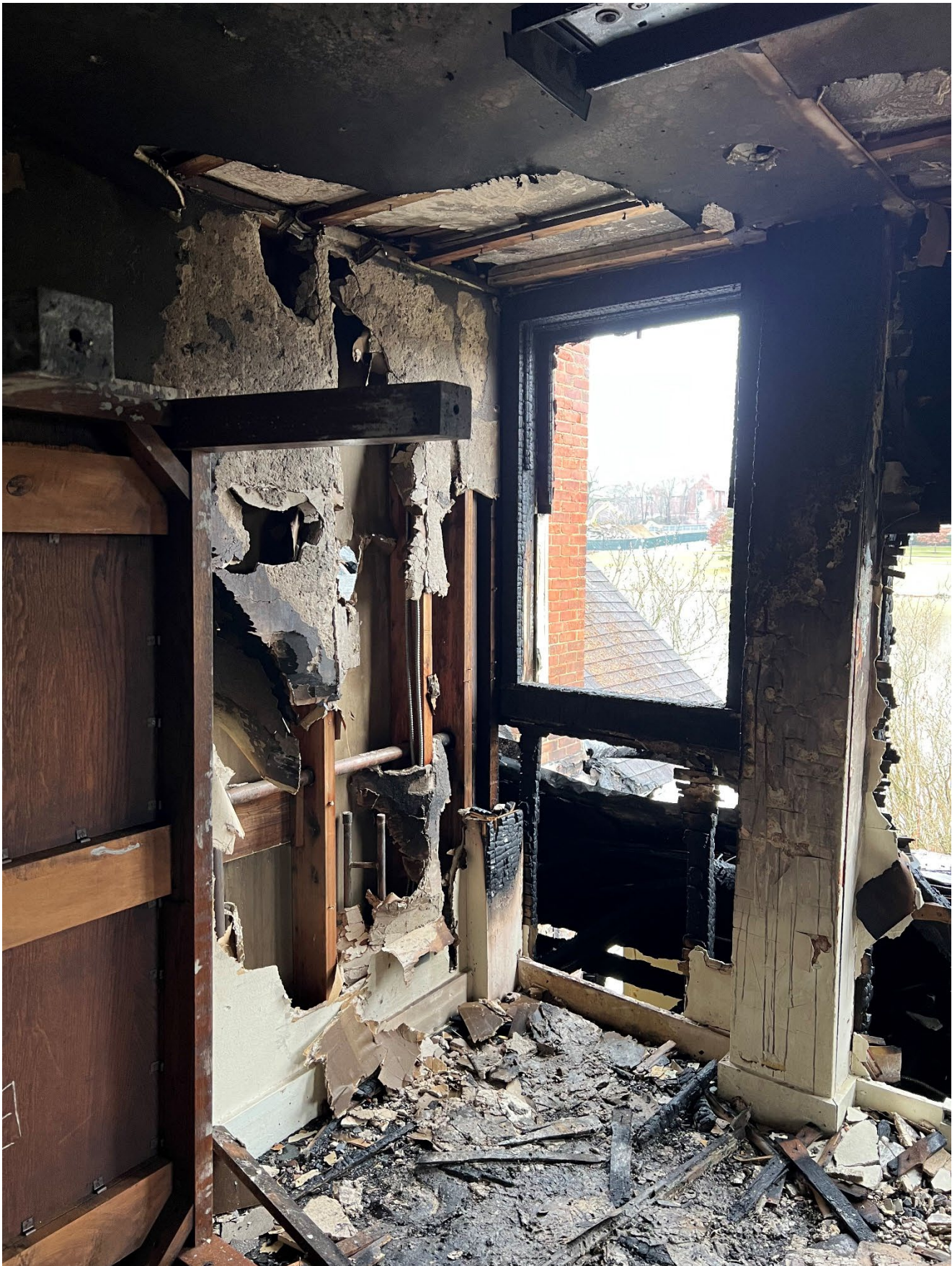
Interior Fire Damage
