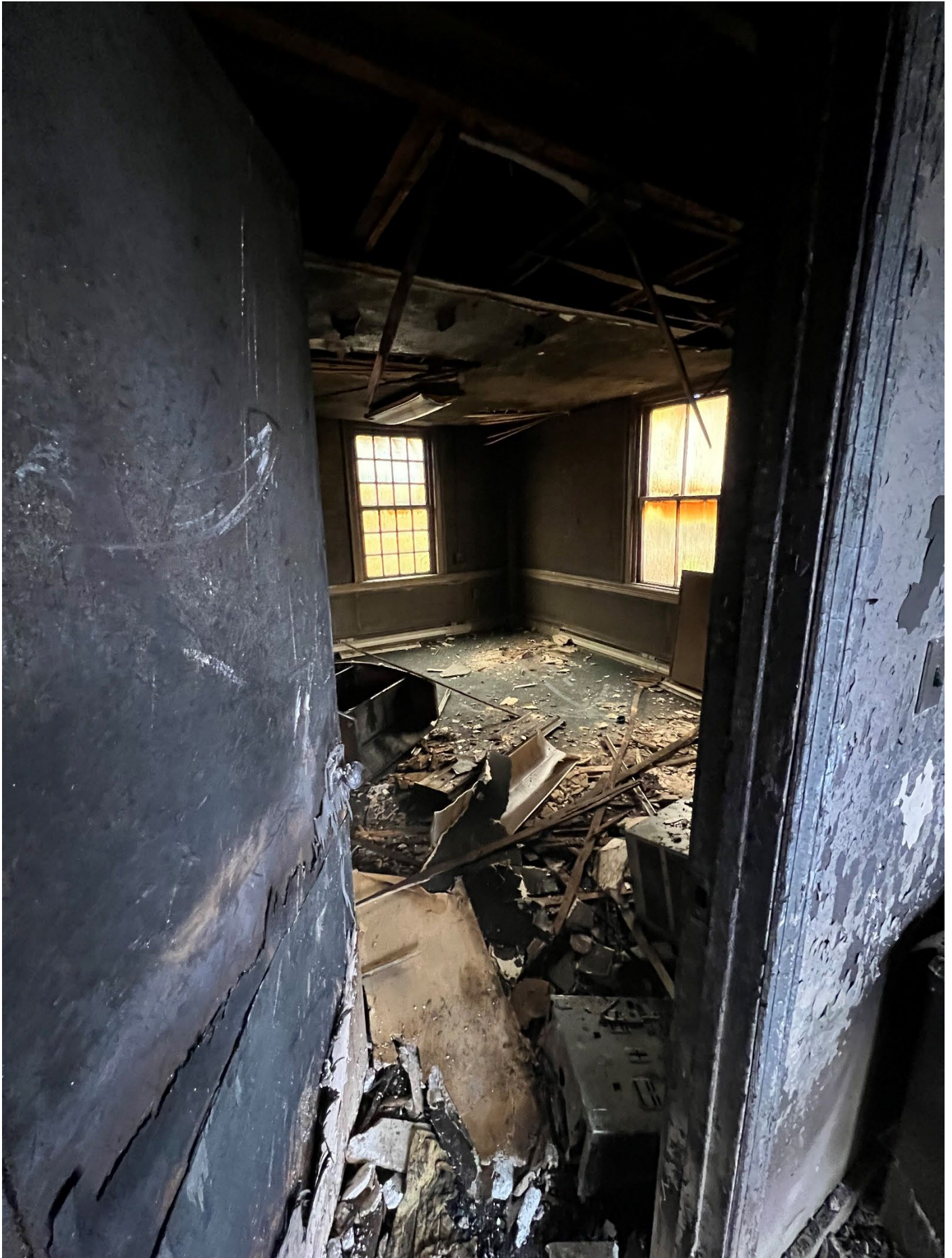
Interior Fire Damage
