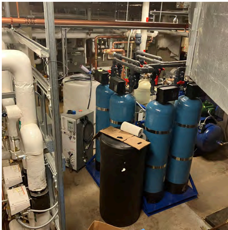
New Reverse Osmosis Water System
