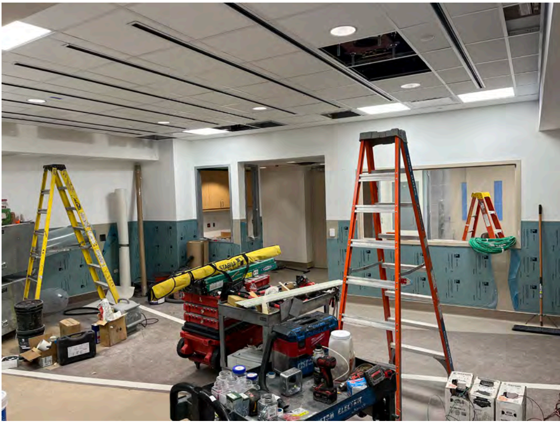
Cath Lab 1 – Procedure Area Looking Toward Entrance and Control Room
