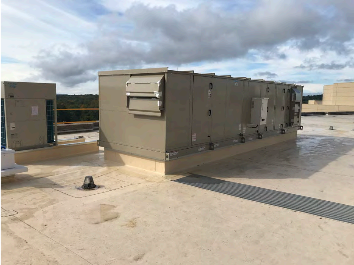
View of new rooftop air handling unit
