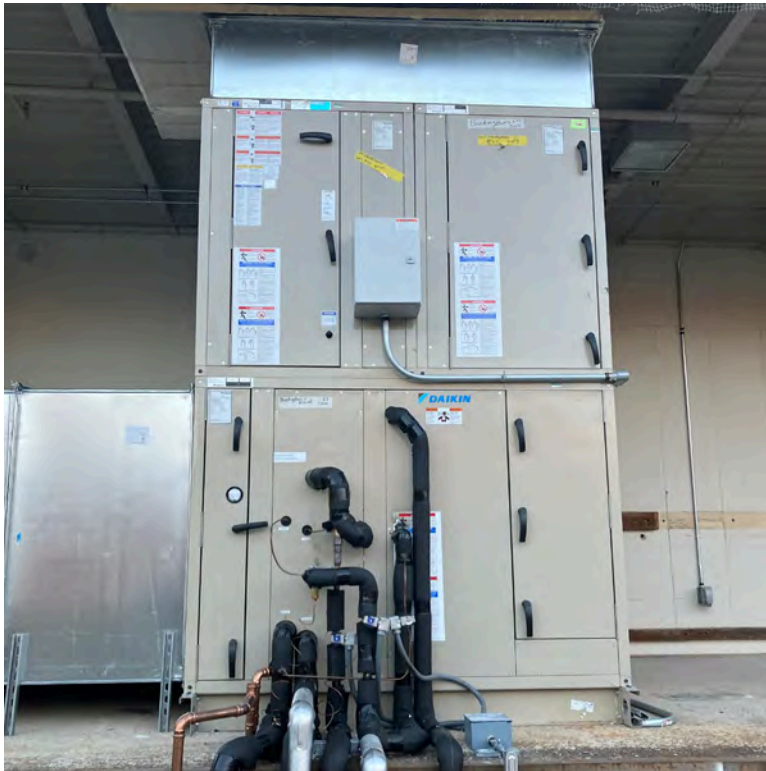
New CRAC Unit
