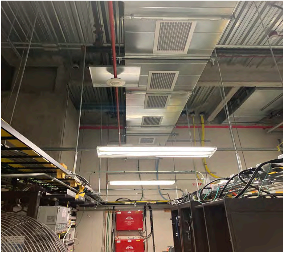
Photo 1 – View of new cooling distribution ductwork
