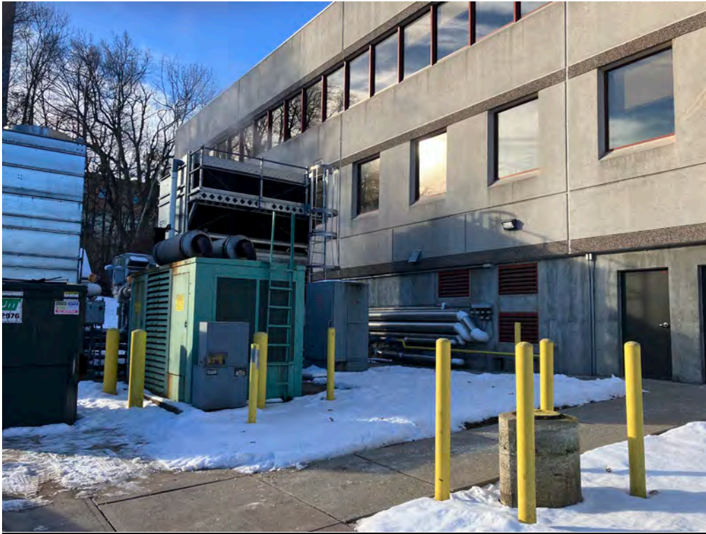
Existing ASB Generator
