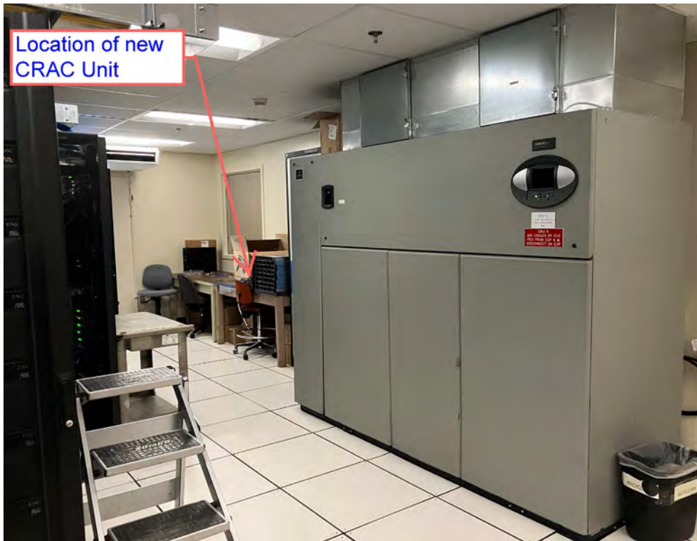
Location of New Data Center CRAC Unit
