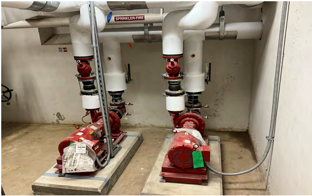
Rogers Hall Dual Temp Pumps
