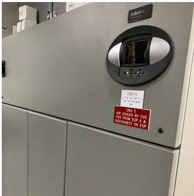
Existing ASB Generator Docking Station
