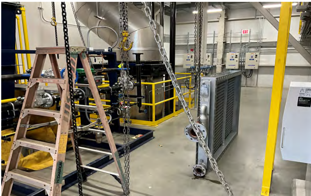
SUP faulty steam coil replacement
