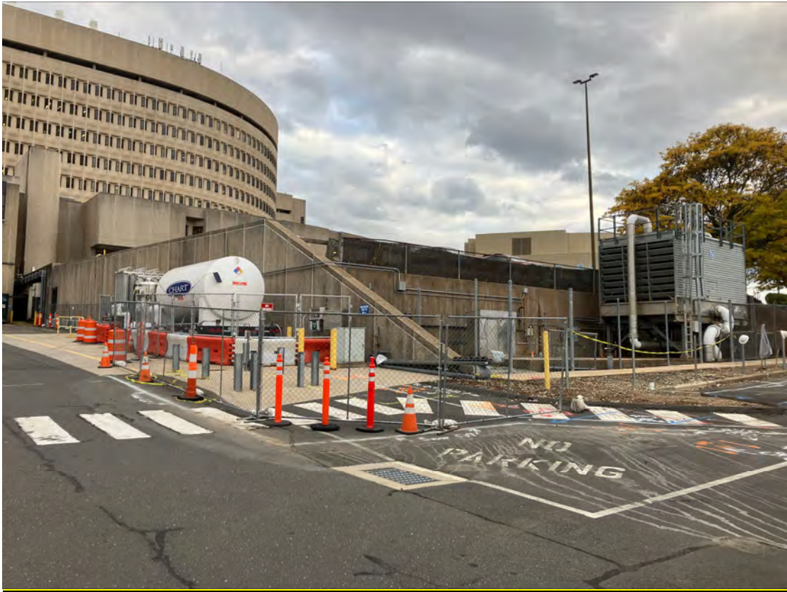
Temporary Liquid Oxygen Trailer at West Dock
