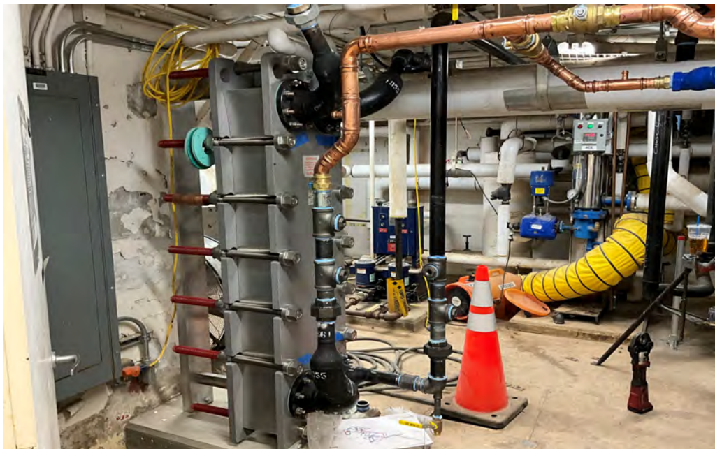
Terry Hall Glycol Chilled Water Heat Exchanger
