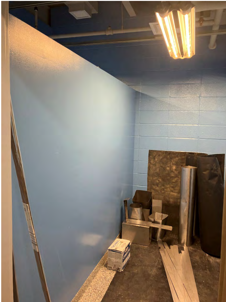
Chemical Holding room
