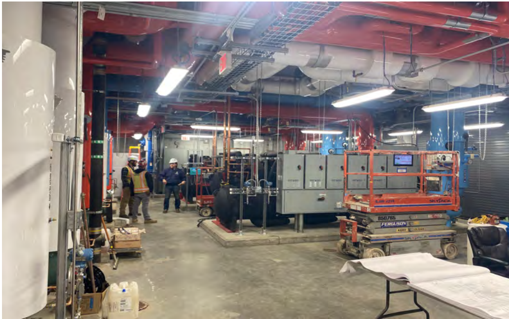
New Heat Recovery Chillers
