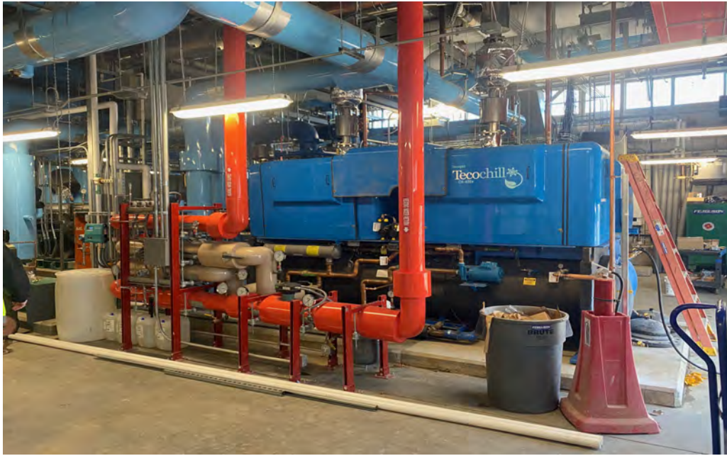
New Gas Fired Chiller
