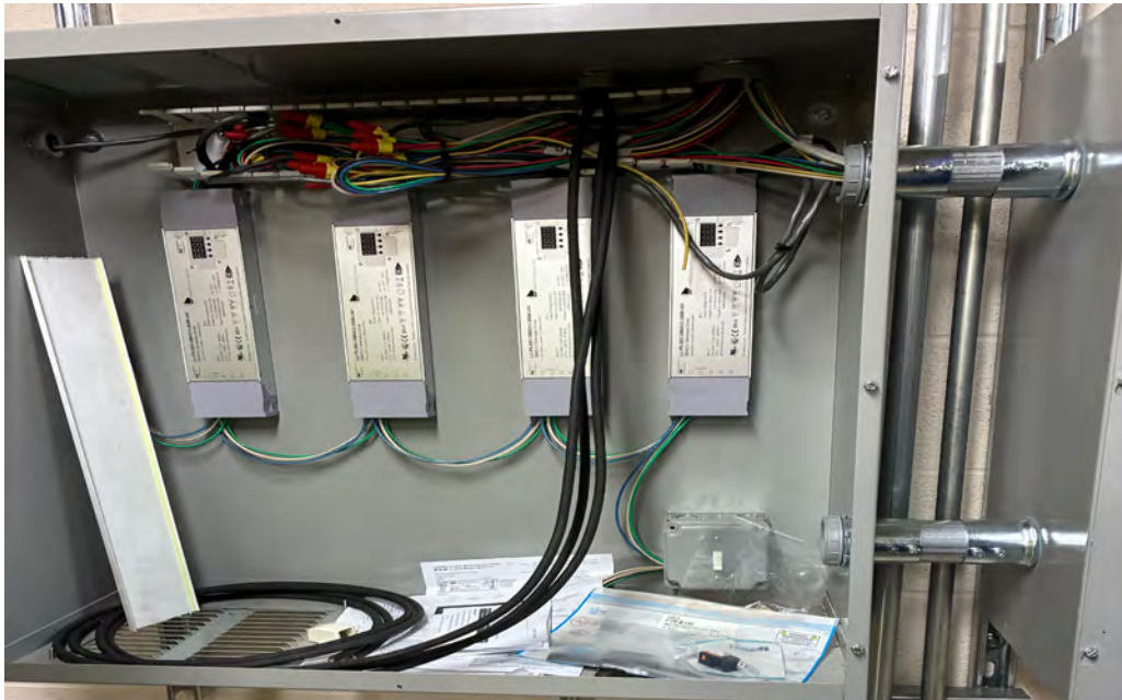
Interior Electrical Box showing Drivers
