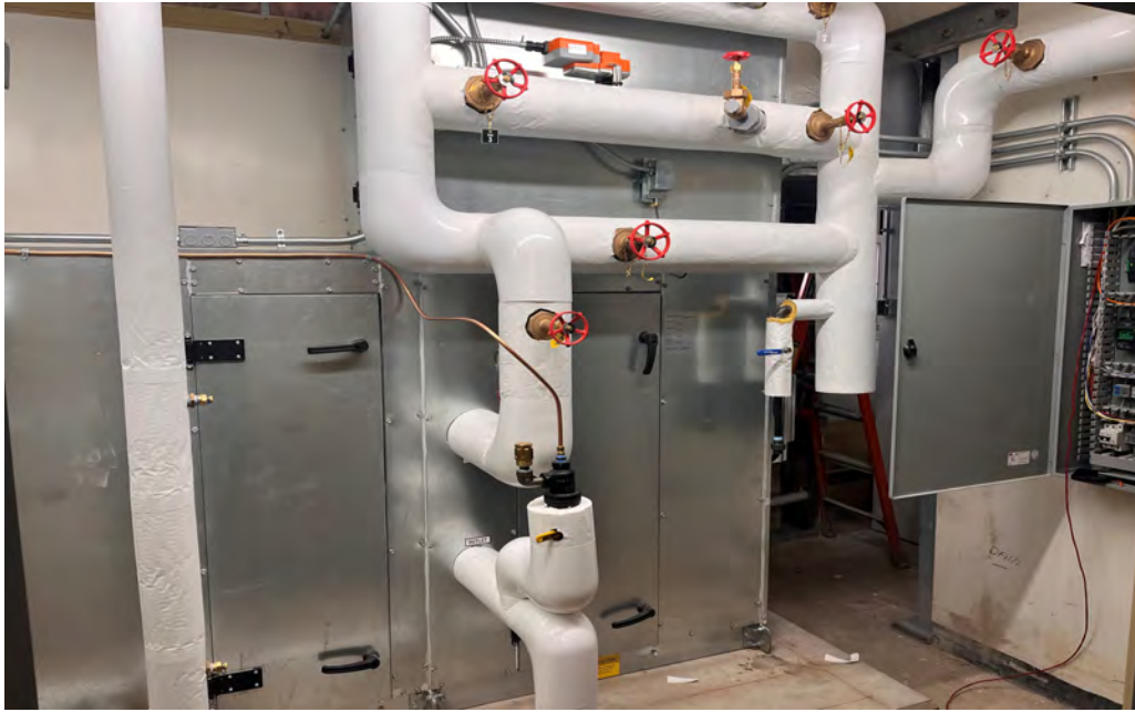
Rogers Hall Make Up Air Unit
