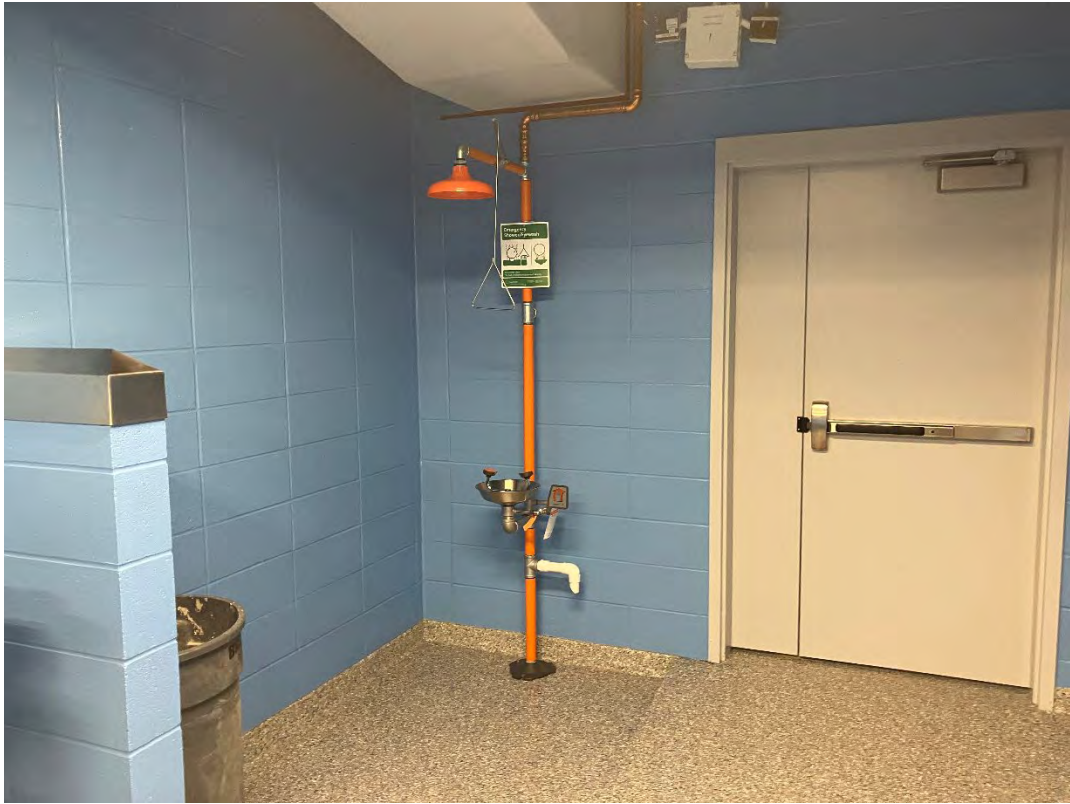
Chemical Holding room
