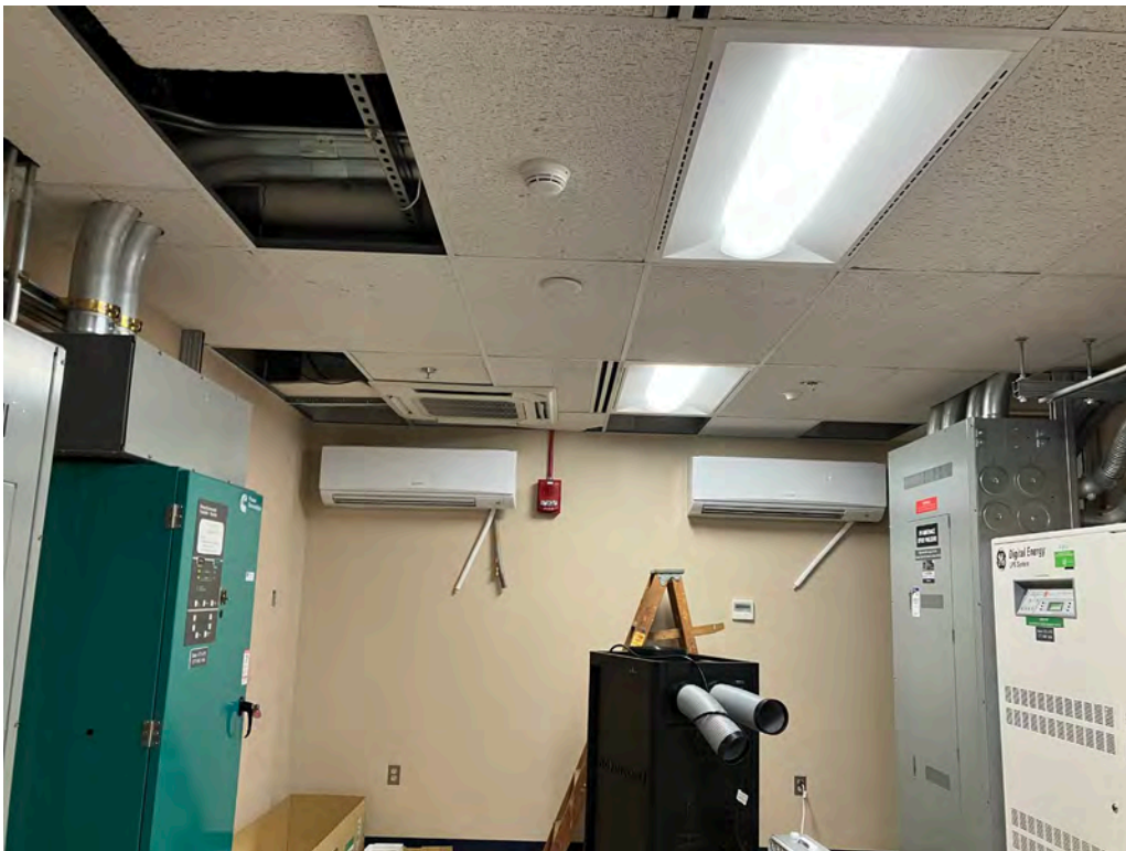
New AC Split Systems in Green UPS Room
