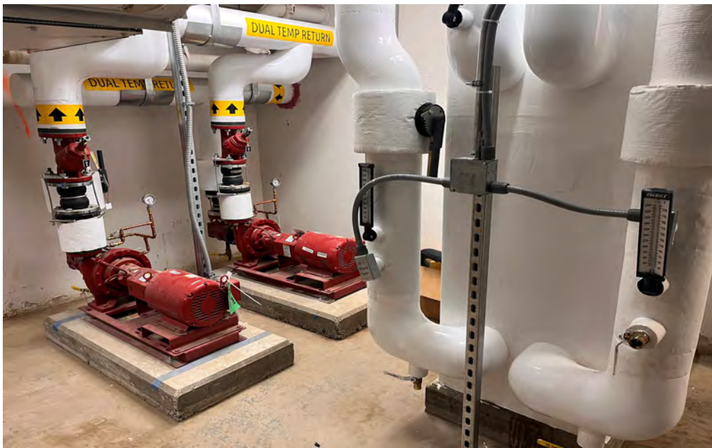
Rogers Hall Dual Temperature Pumps and Heat Exchanger
