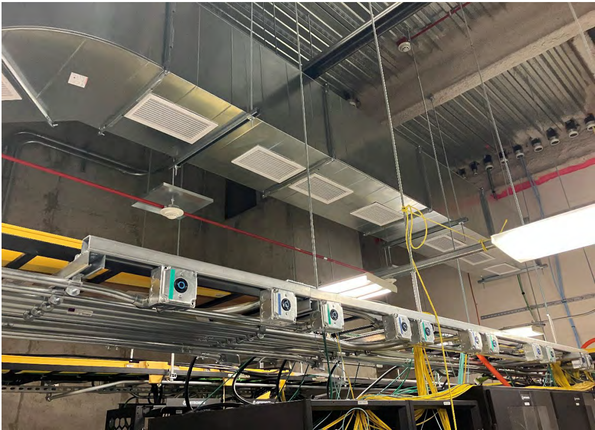
View of cold air supply distribution ducts.
