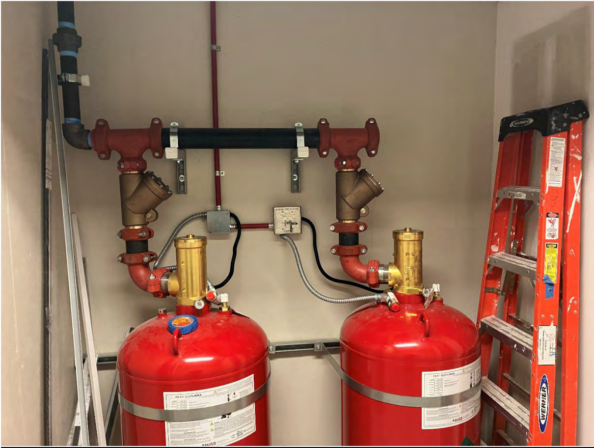
View of new clean agent storage room & tanks
