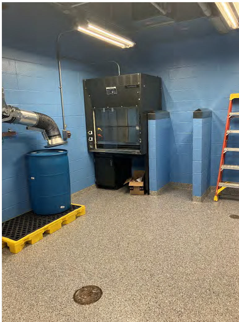
Chemical Holding Room / Fume Hood
