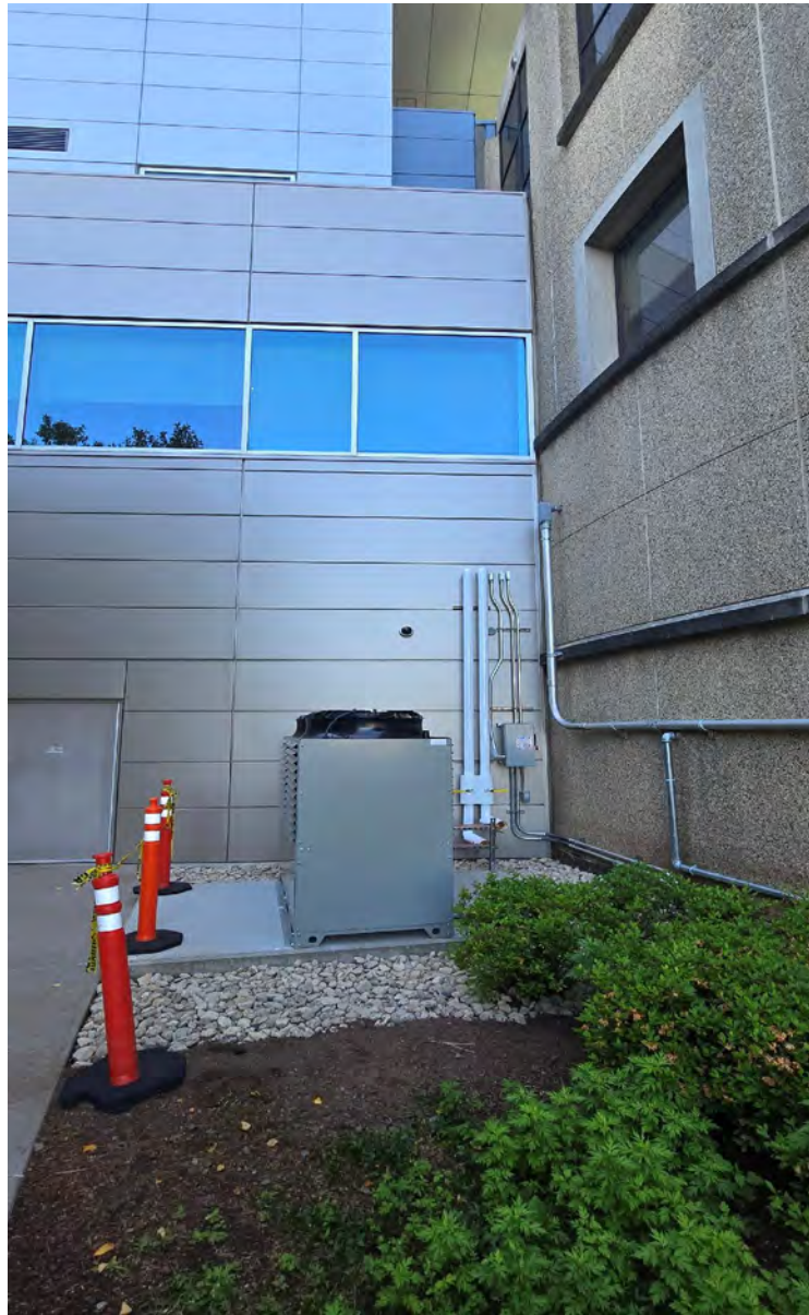
New Dedicated Chiller for MRI
