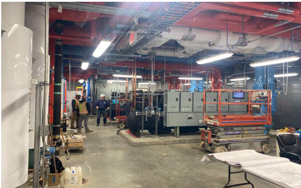
New Heat Recovery Chillers
