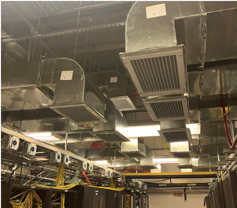
View of cold air supply distribution ducts.
