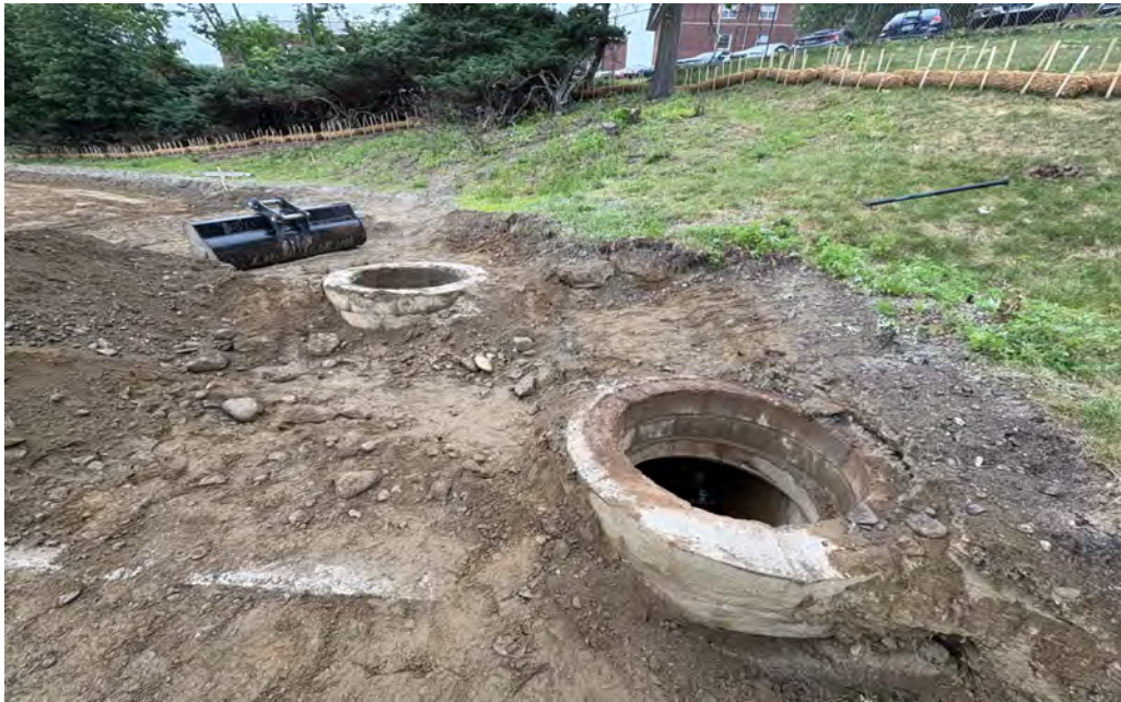
Undocumented Steam Vault discovered during Demolition
