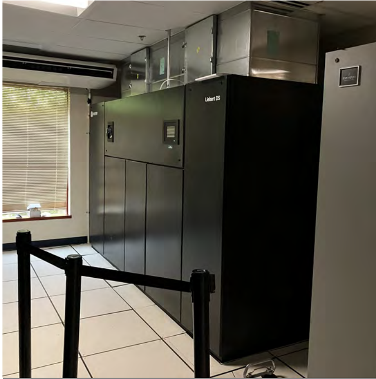
New CRAC Unit 6 installed in the Data Center
