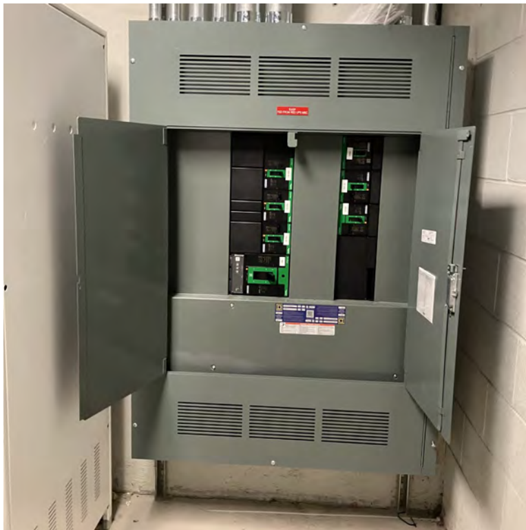
New Emergency UPS Distribution Panel (EUDP) in Red UPS Room
